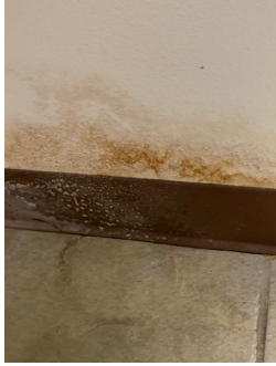
Some plumbing repairs are needed in our bathrooms
