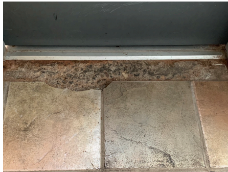
and missing threshold
