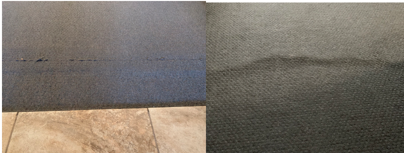
Cracks under our carpeted floor which are tripping hazards
